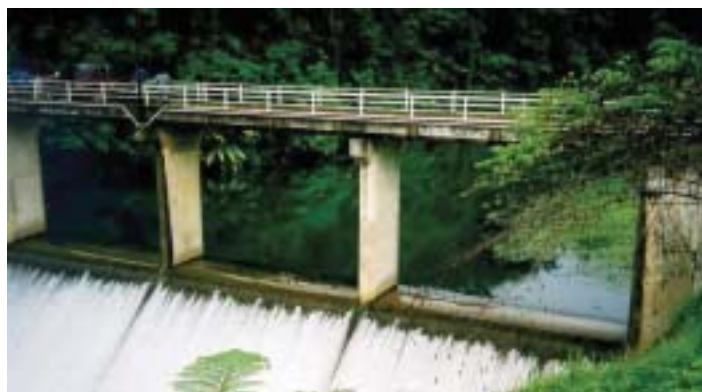
Hydropower dam, Espiritu Santo, Vanuatu
