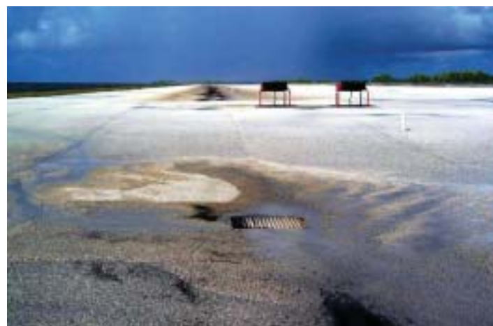
Runway rainwater catchment, Majuro, Marshall Islands
